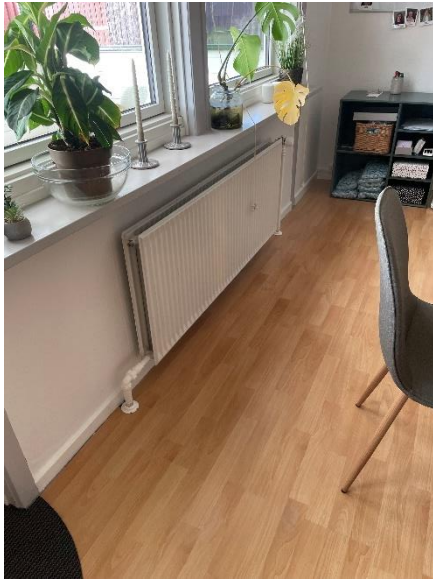
Radiator i rum ud mod terrasse, 2 strengs system
