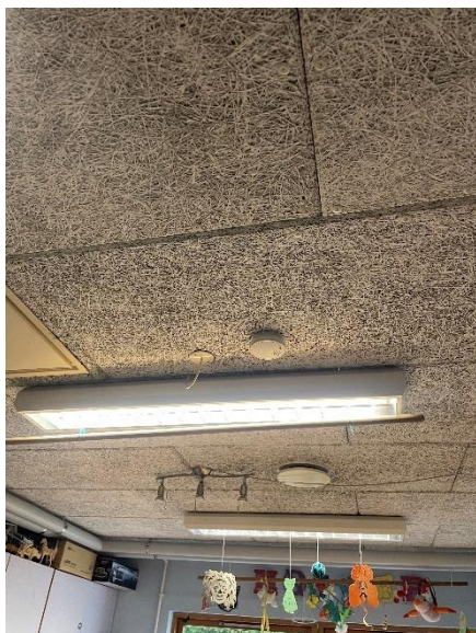
Brandalarm i loft.
