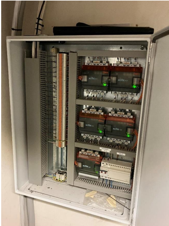
CTS understation i varmecentral
