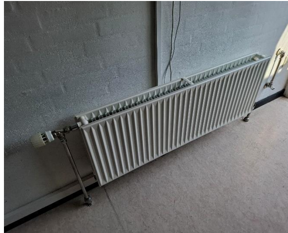
Radiator i stuen
