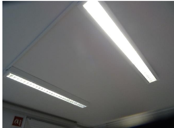
LED armaturer i stueetagen
