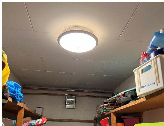
Armatur i depot
