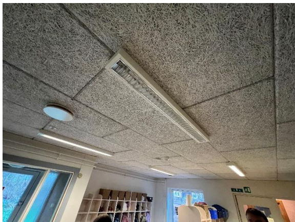
Armaturer i stueetagen
