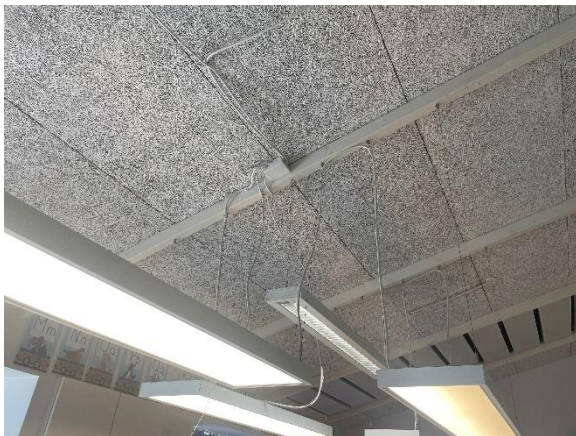
Ulovlig kabellus mellem to Led armaturer
