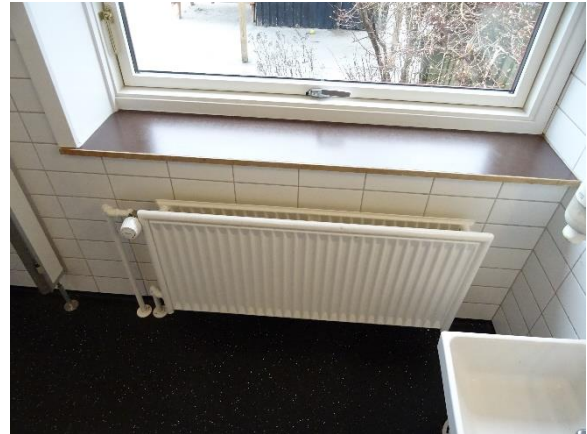
Radiator i toiletrum
