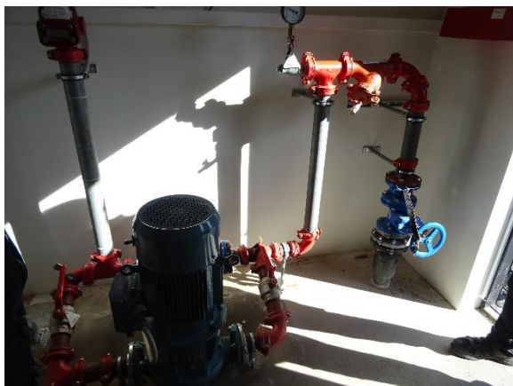
Sprinklerpumpe i central
