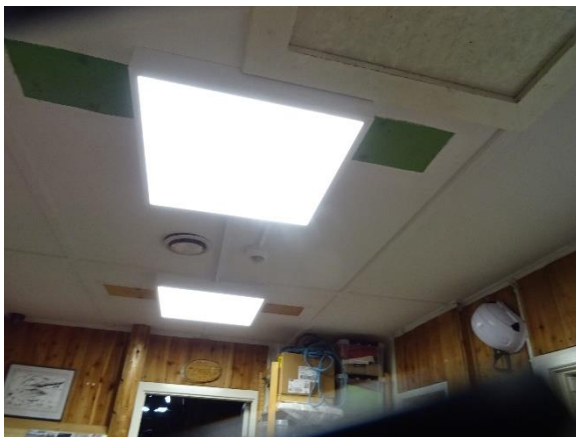
LED paneler forrum
