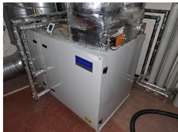
Ventilationsenhed for procesudsugning.
