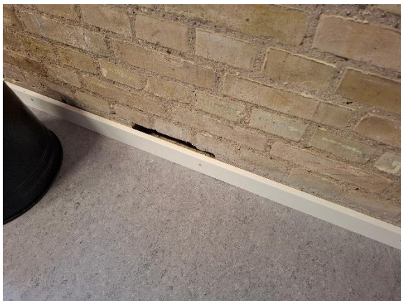
Manglende sten bag fodpanel.
