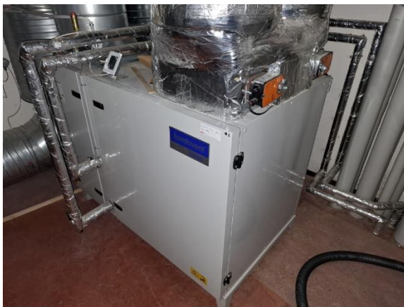
Ventilationsenhed for procesudsugning.
