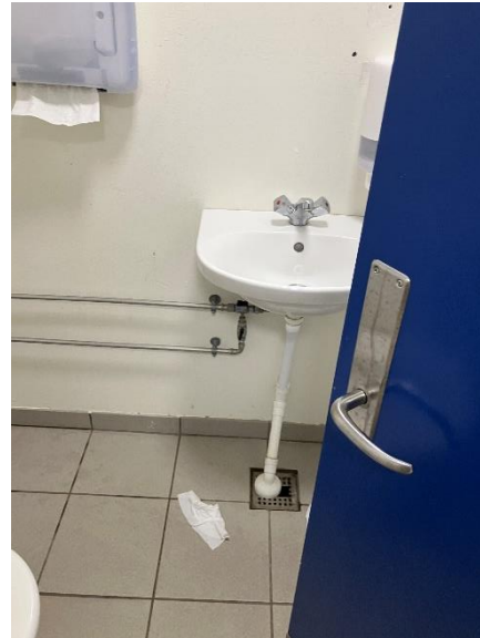
Mangler rottesikret rist
