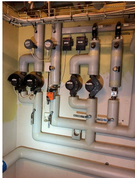
Fordelingspumper i varmecentral
