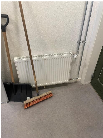
To strengs radiator i bad/omklædning
