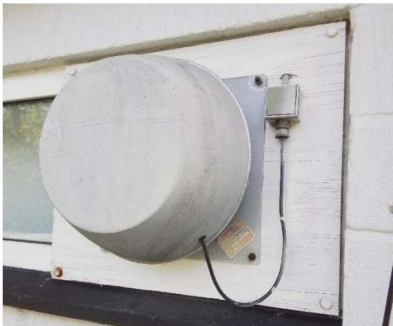
Ventilator i facade
