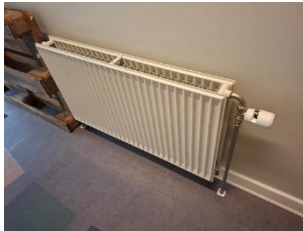
Nyere to-lags radiator.
