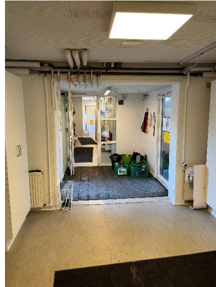
LED paneler i gangareal
