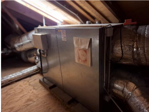
Ventilationsaggregat i loftrum
