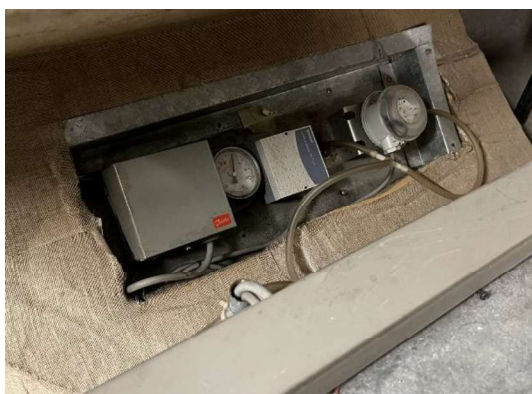
Automatik for ventilationsaggregat
