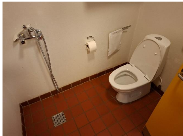
Toilet/bad for personalet
