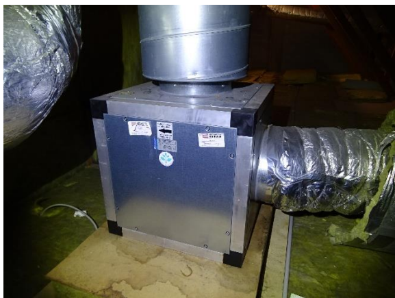
Boksventilator for toiletter
