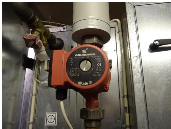
Pumpe ventilationsvarmefflade, manuelt trinstyret
