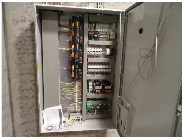
Honeywell undercentral i varmecentral
