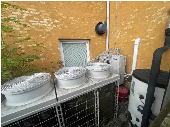
Varmpumpe ydre installation i bygn.20
